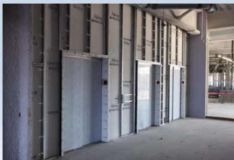
Still wrapped in plastic the elevators sit ready for use as construction continues. Two separate banks of elevators are designed to keep visitor flow and patient flow separate.
