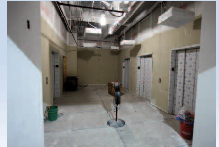
A bank of elevators at the new hospital.
