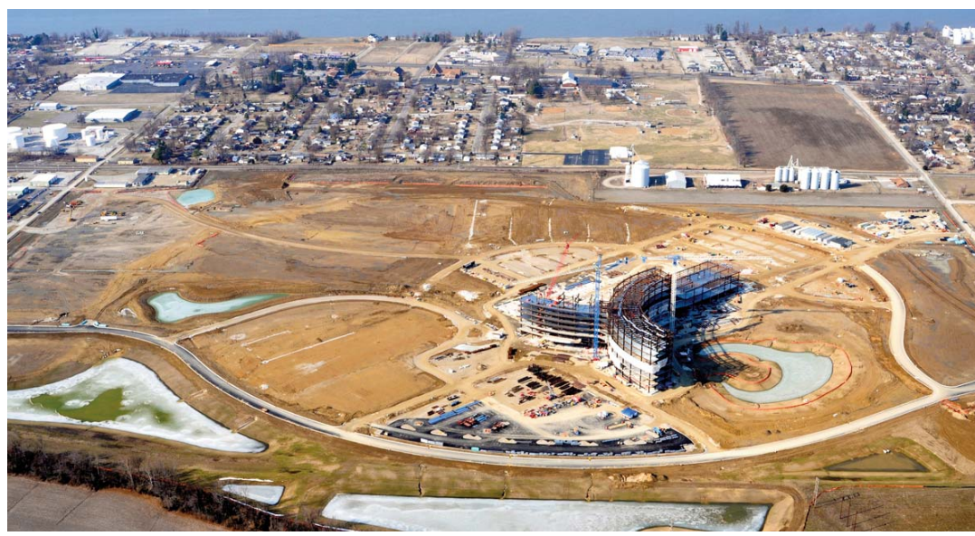
Steel work is almost complete and on Friday the highest piece of steel will be put in place as part of the Topping Out ceremony.
