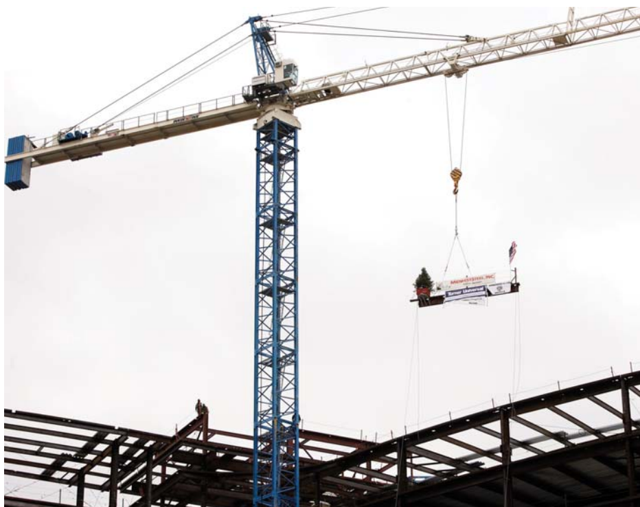
The highest piece of steel was raised into place on Friday, February 25th. The beam was placed on the top floor of the structure, which sits 150 feet above the ground.
