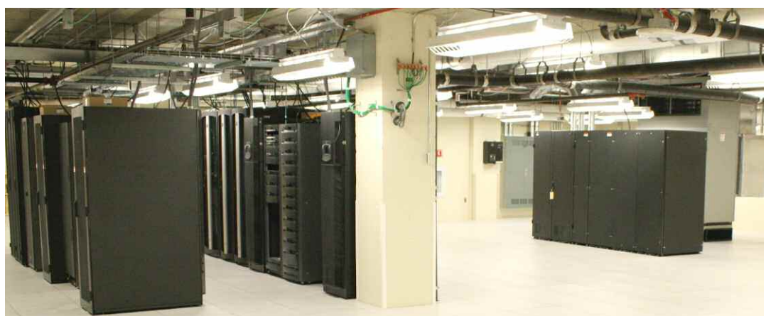
Room to grow; the new data center at OMHS houses all of the organization's drives and information necessary to run the hospital and help employees do their job faster.
